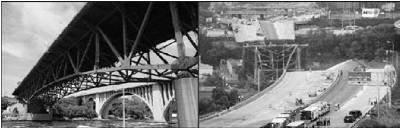
Figure 1. The I-35W Mississippi river bridge - Before and after failure
